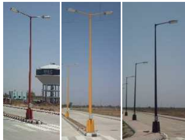
Installation of GRP Poles in Red, Yellow & Blue colours at Gujarat Industrial Development Corporation, Vadodara
