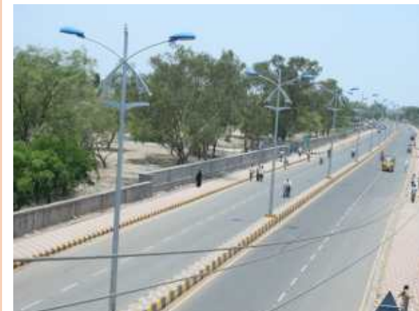
9 mtr Octagonal Pole with decorative bracket installed at Bellary City Corporation
