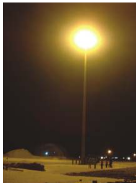
Complete erection of 40m (22 nos.) and 50m (4 nos.) masts at ICTT – Kochi.
