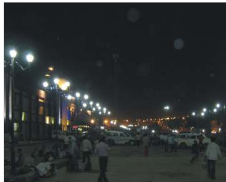
The first prestigious Supply, Installation, Testing and Commissioning of Decorative Poles executed by Patna Branch for Rajendra Nagar Terminal. Value: Rs. 30 Lakhs.
