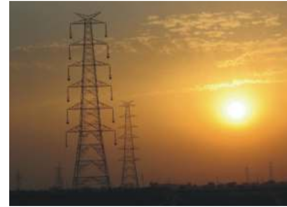
400 kV Double Circuit Line at Vijaywada.
