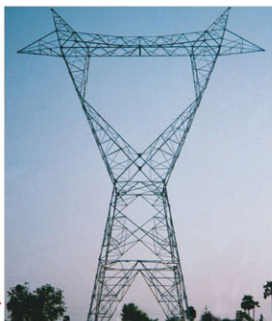
Single circuit Transmission Line tower for Hyderabad-Karnool Gattil line
